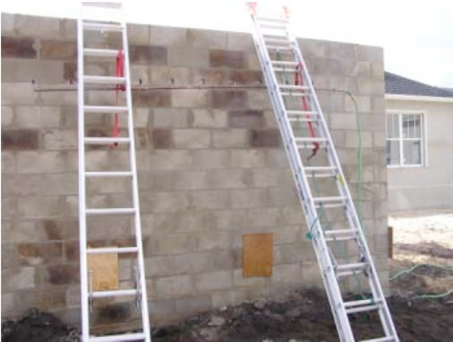
Photograph 54: Spray Rack Without Induced Pressure Difference
