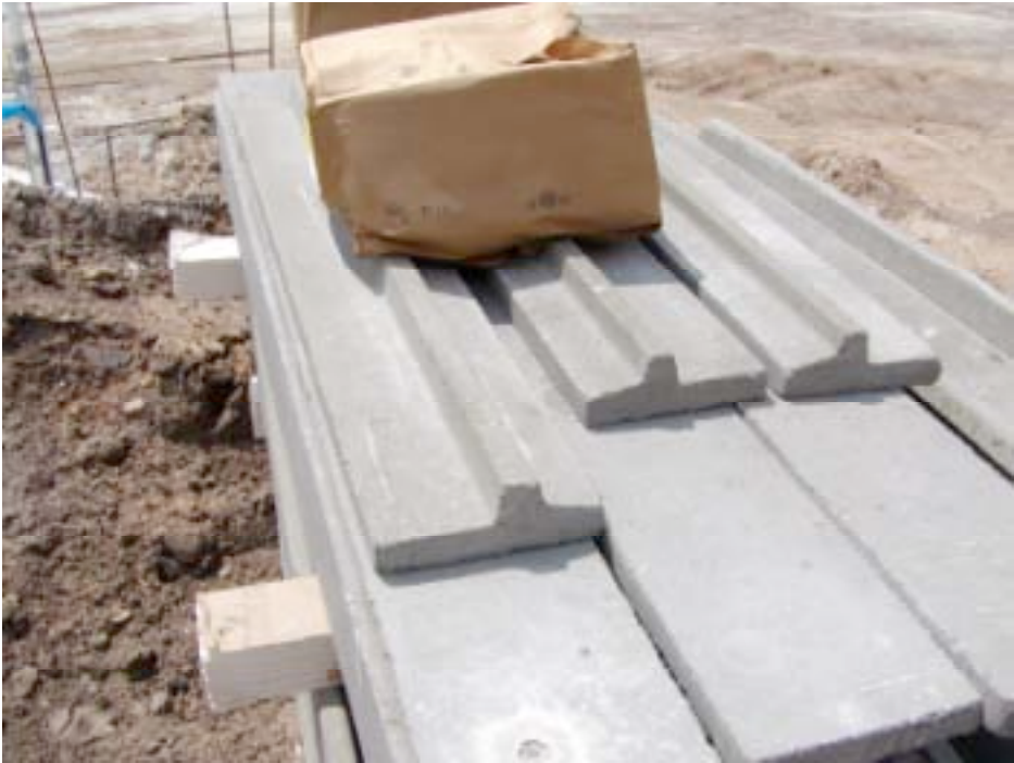
Photograph 27: Precast Sill With Illogical Attachment Rib
