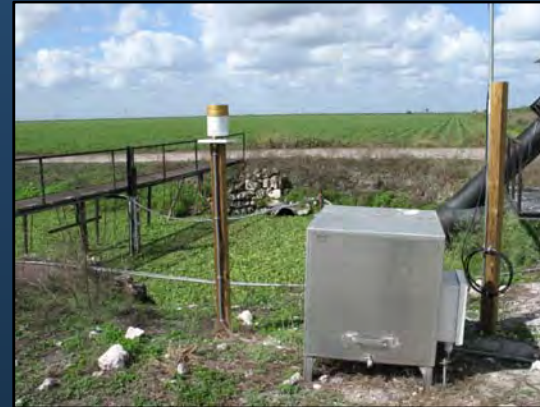
Rain gauge, 1/2 to 1-inch rainfall detention
