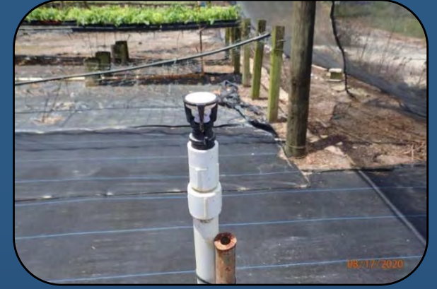
Replacing traditional rotary sprinkler with Mini-Wobbler, reduces water and energy use
