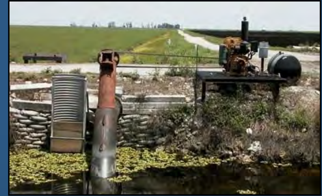
Internal pumps to reduce off-farm drainage
