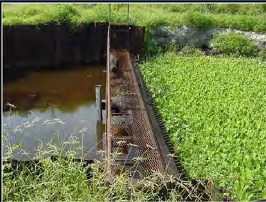
Aquatic weed racks to capture particulates
