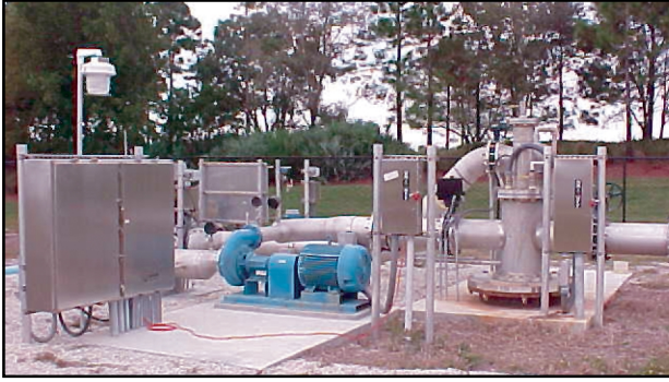
Figure 6-5 Raw Water Booster Pump
