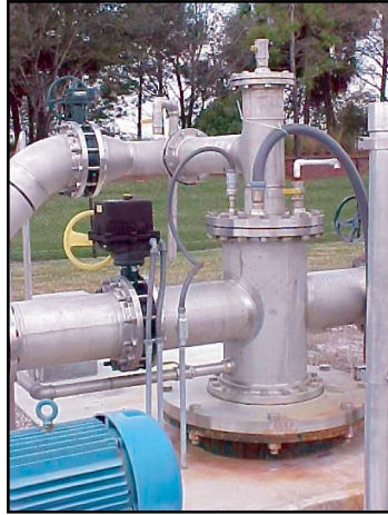
Figure 6-3 3W ASR Wellhead
