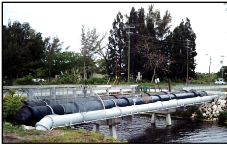
Figure 6-19 Membrane Concentrate Line between WTP 3 and SRWRF
