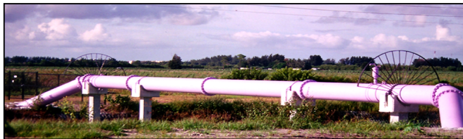
Figure 6-9 SRWRF Reclaimed Water System Distribution Piping
