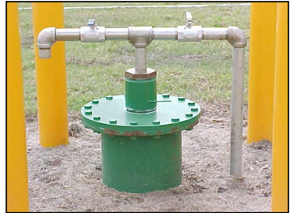
Figure 6-4 3W Monitor Well
