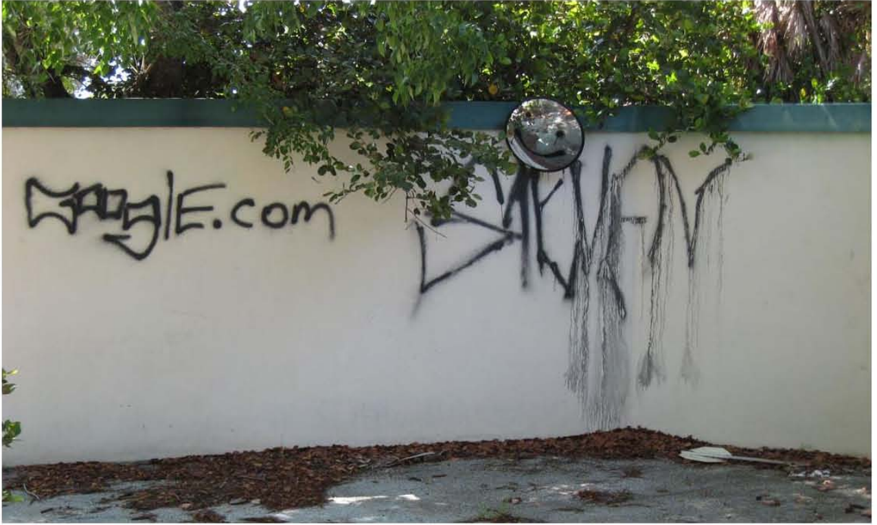
Examples of Vandalism
