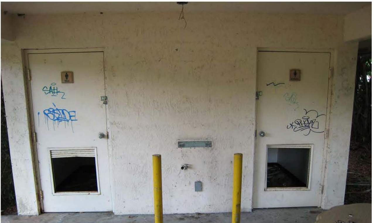
Examples of Vandalism
