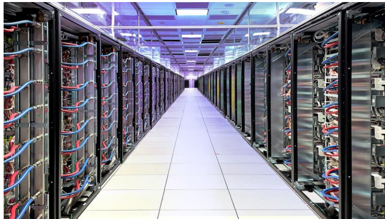
Figure 2 – Submer Company Direct Liquid Cooling System
