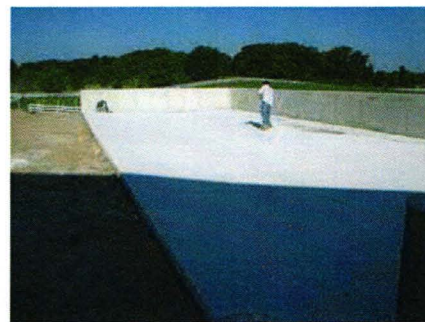
Figure 2. Concrete manure storage pad
