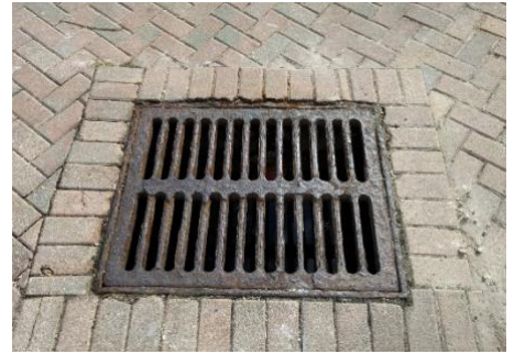
Figure 1-25. A stormwater inlet in Delray Beach. Photo by Anna Leitschuh, Collective Water Resources.
