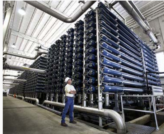
Floridan brackish ground water wells and treatment plant
