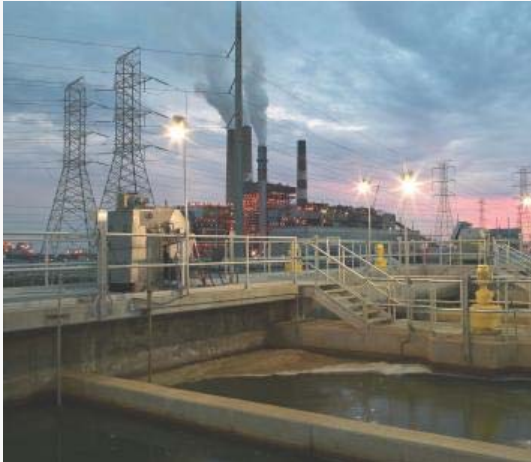
Seawater desalination treatment plant
