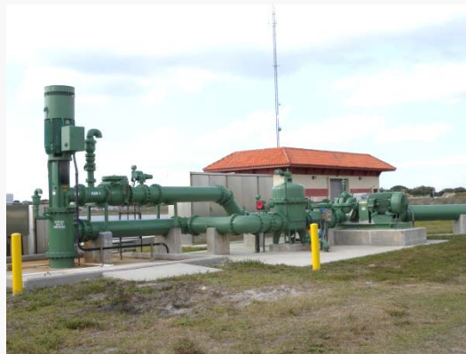
Aquifer Storage and Recovery Well
